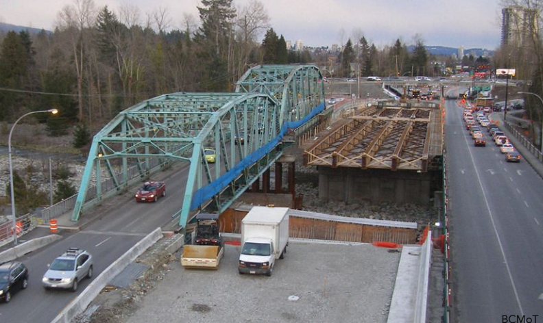
▲ New steel girders being launched from the Capilano River's east bank, over the river pier and closing in on west abutment.
